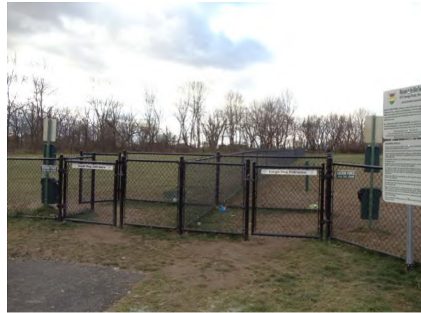
Compaction and erosion at point of entry into fenced areas.
