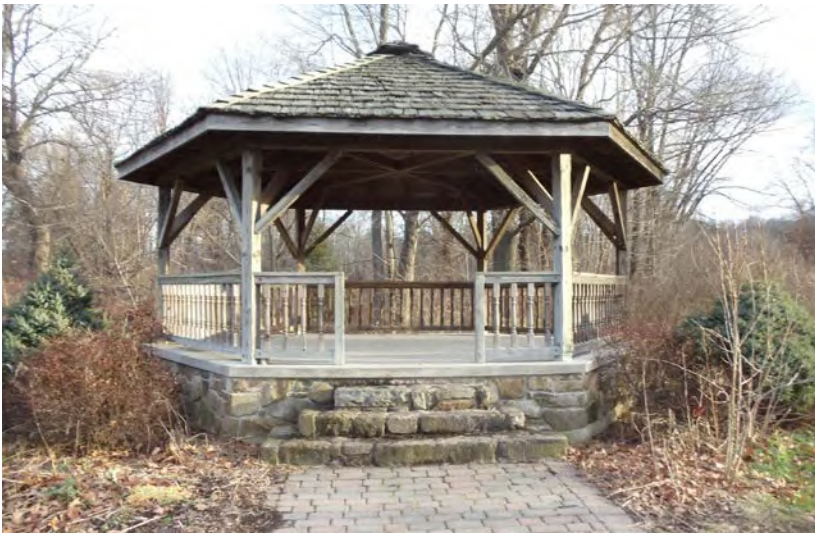
Gazebo – Note the facility is not ADA accessible.
