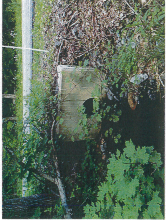
Photo 19 – Outfall 14-A – 15-inch N-12 plastic pipe with concrete endwall along an unnamed tributary to Hokendaqua Creek.
