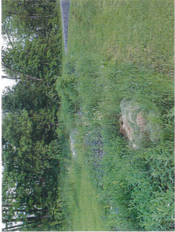
Photo 9 – Outfall 5-B – Seepage from basin floor into rock-lined channel leading to Dry Run.
