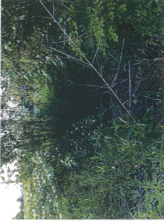
Photo 14 – Outfall 10 – 15-inch N-12 plastic pipe leading to headwater wetlands to Dry Run.
