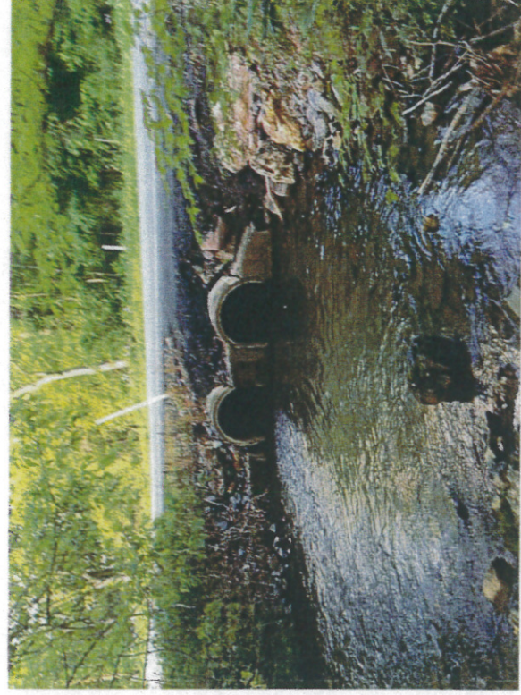
Photo 20 – Outfall 14-B – 2x30-inch reinforced concrete pipe with concrete endwalls along an unnamed tributary to Hokendaqua Creek.
