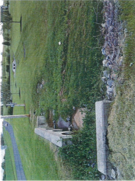
Photo 5 – Outfall 3-B – Grassed swales leading to Outfall 3 inlet from the recently developed Wayne Grube Park.
