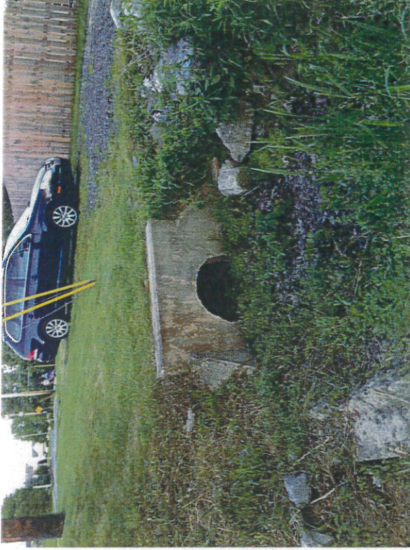
Photo 6 – Outfall 4 – 30-inch N-12 plastic culvert with concrete endwall and rip-rap outlet protection.
