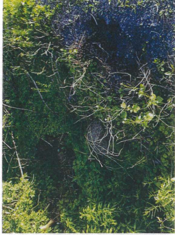
Photo 16 – Outfall 11-B – 24-inch reinforced concrete pipe leading to headwaters of Dry Run.
