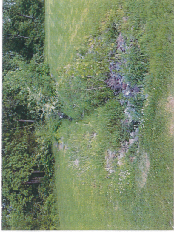
Photo 10 – Outfall 6 – Rock-lined channel to Dry Run from corrugated outlet pipe from stormwater basin.
