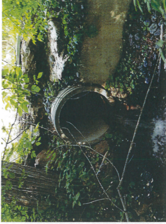
Photo 18 – Outfall 13 – 30-inch reinforced concrete pipe with quarry block endwall to an unnamed tributary to Hokendaqua Creek.
