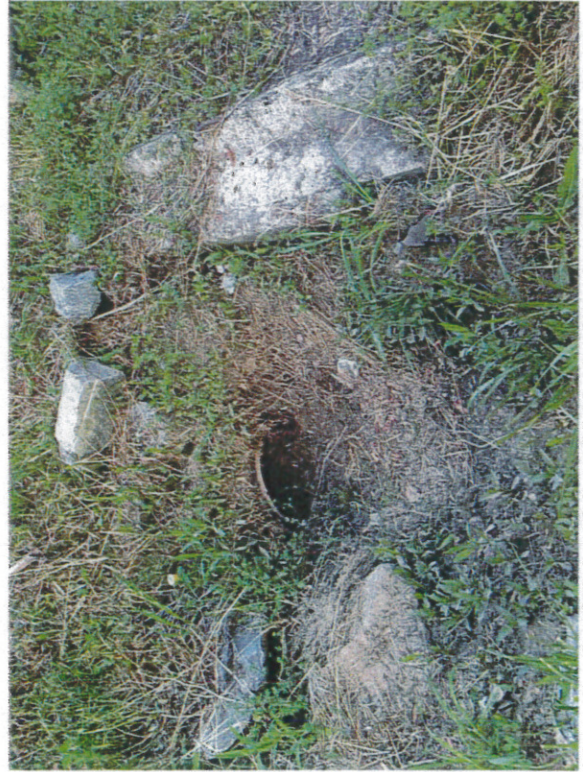
Photo 7 – Outfall 4 – 15-inch N-12 plastic culvert with rip-rap outlet protection.
