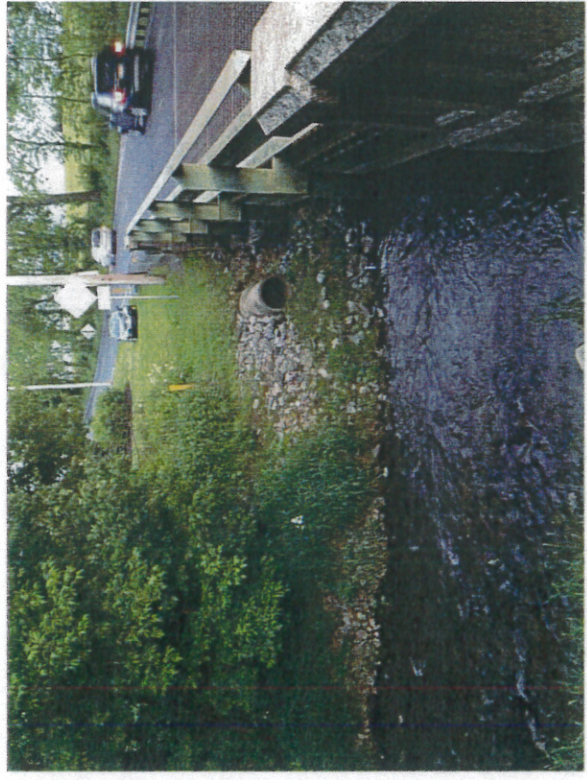
Photo 1 – Outfall 1-A – 15-inch reinforced concrete pipe and 15-inch N-12 plastic pipe to Catasauqua Creek.
